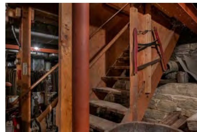
Basement Lacks ADA accessibility Keep existing function as collections storage and general building maintenance support
