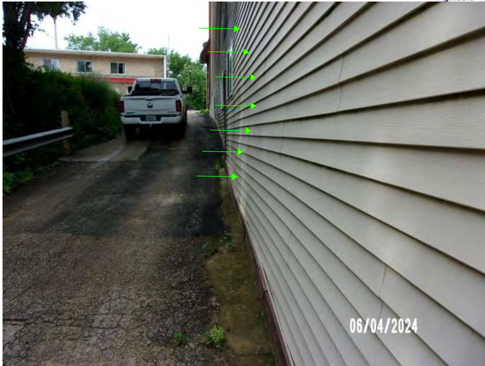
Photo 1 – East wall bowing in above grade
