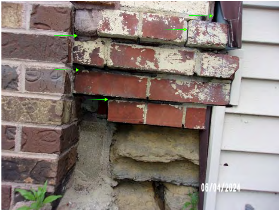
Photo 6 - Loss of mortar at the corbel near the ground on the southeast corner of the building
