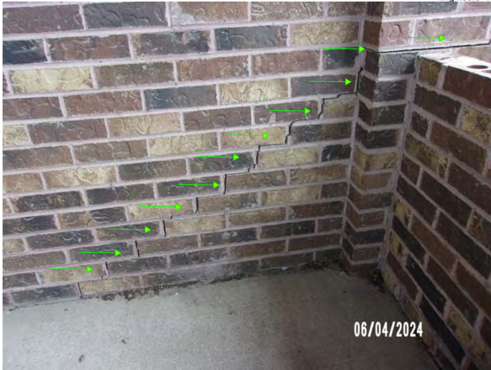
Photo 9 – Crack in south brick wall
