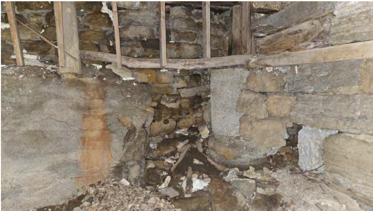
Photo of SE corner of lower basement showing crumbling stone foundation, timber floor support system and concrete concrete wall poured against stone foundation.
