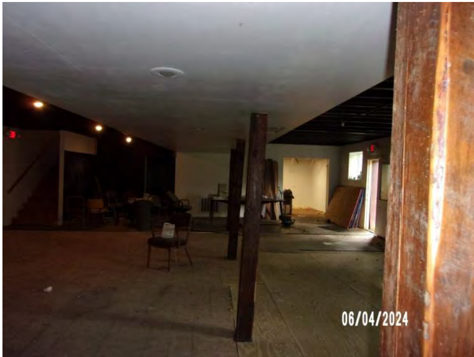
Photo 12 - Interior columns lean to the east significantly
