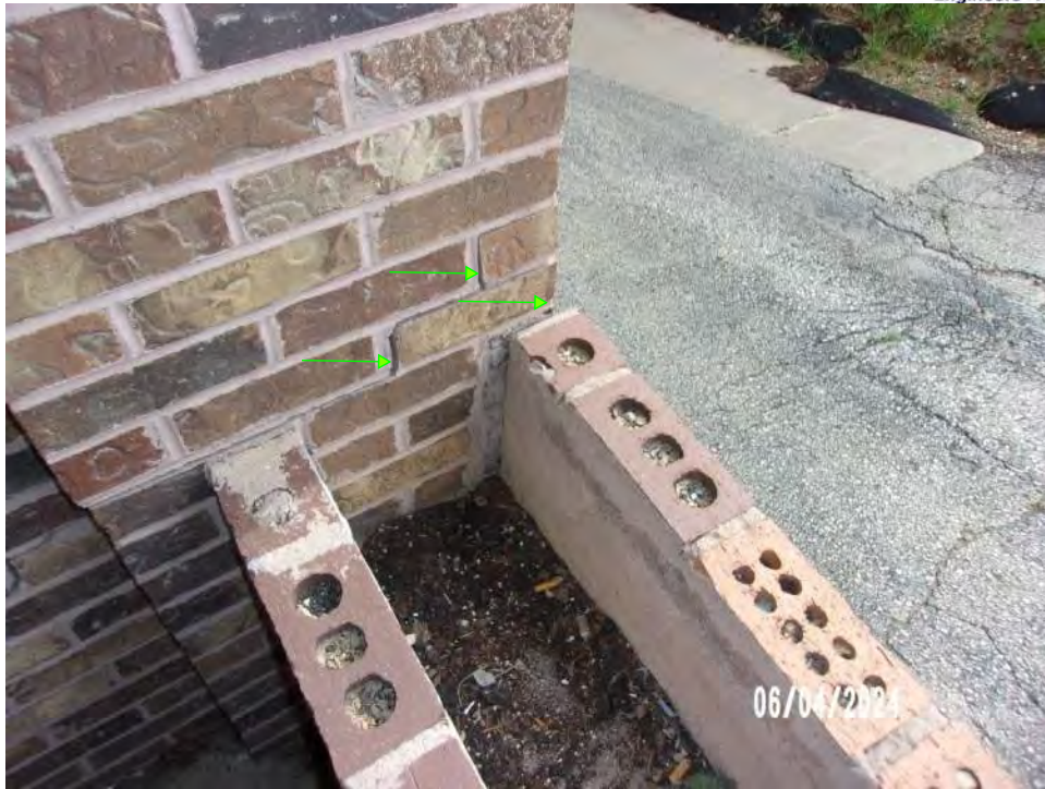
Photo 7 - Brick planter wall leaning east
