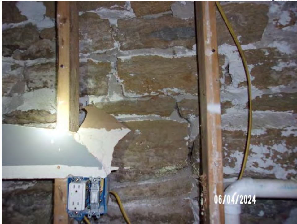
Photo 13 – Crack in south stone foundation wall
