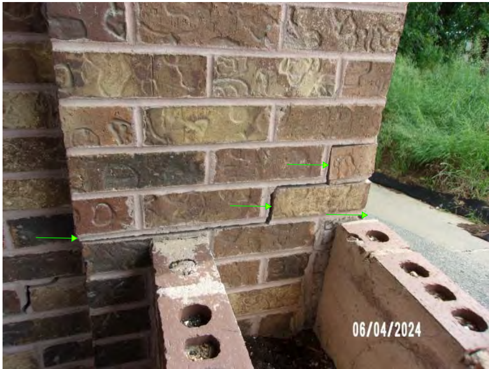
Photo 8 - Crack in south brick wall
