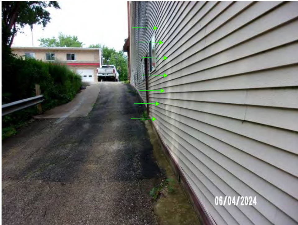
Photo 2 – East wall bowing in above grade
