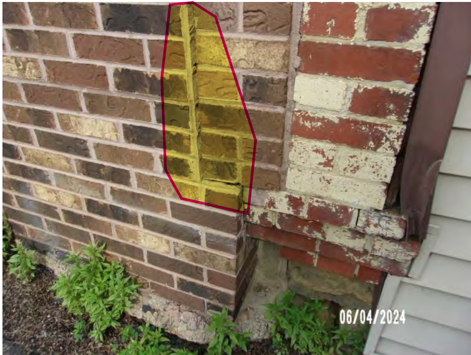
Photo 4 – Brick planter wall leaning east
