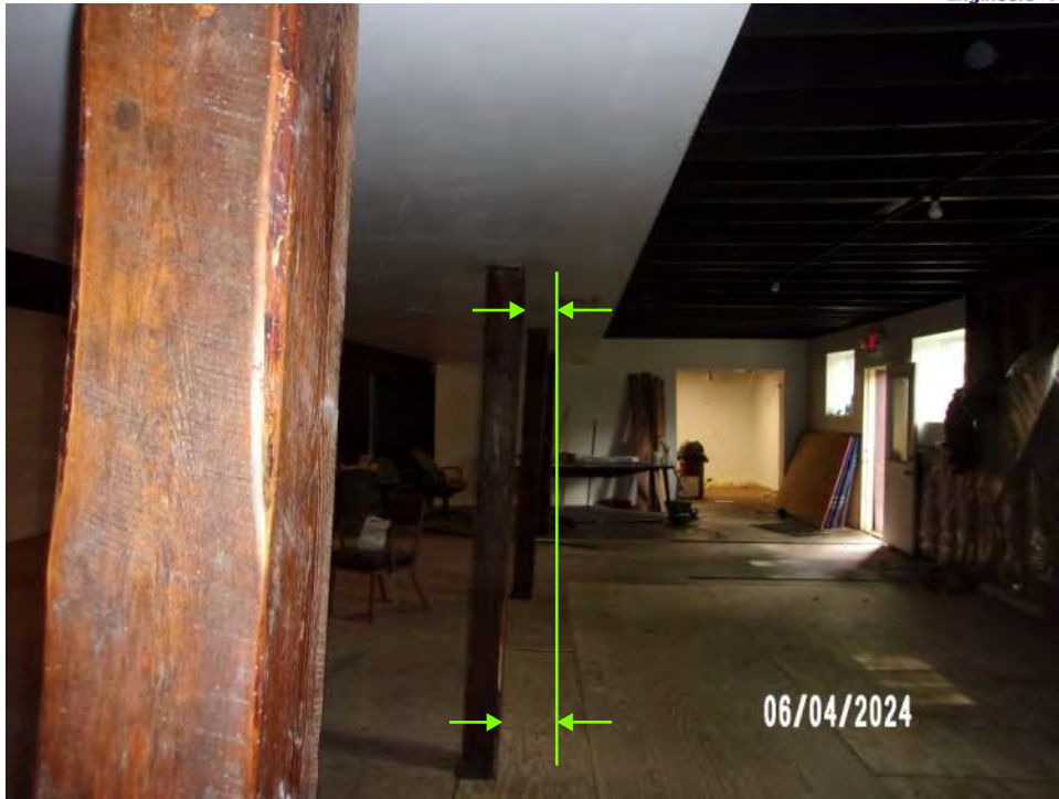
Photo 11 – Interior columns lean to the east significantly
