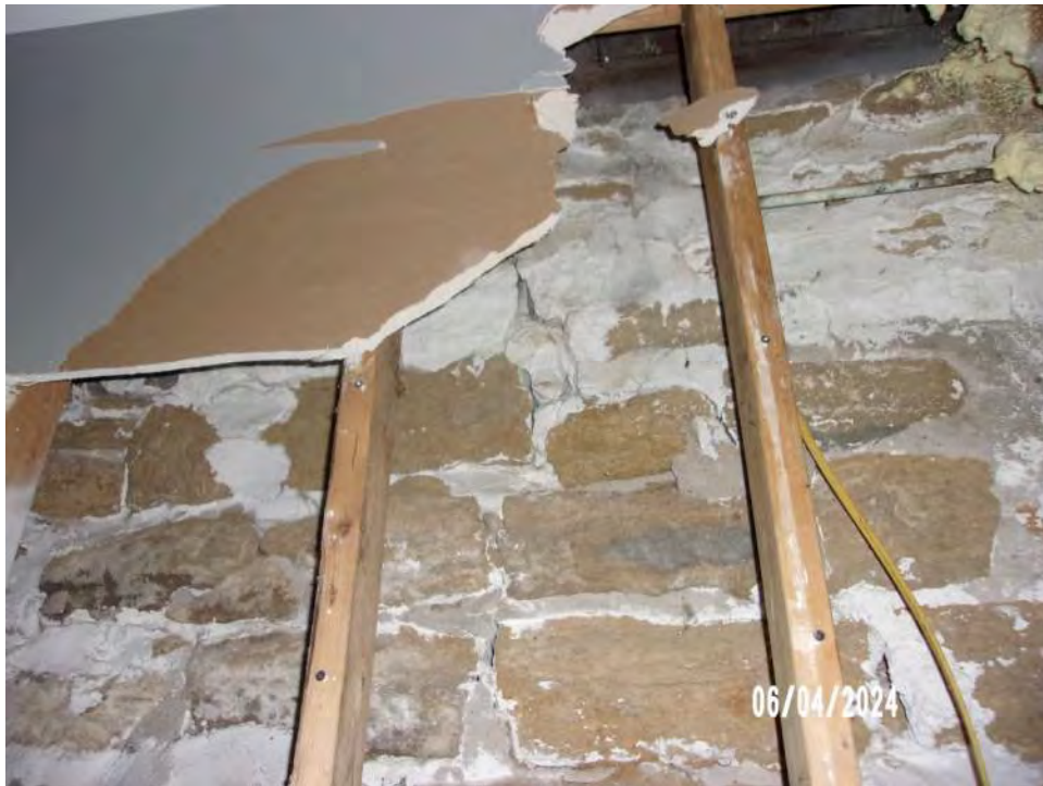
Photo 14 – Crack in south stone foundation wall
