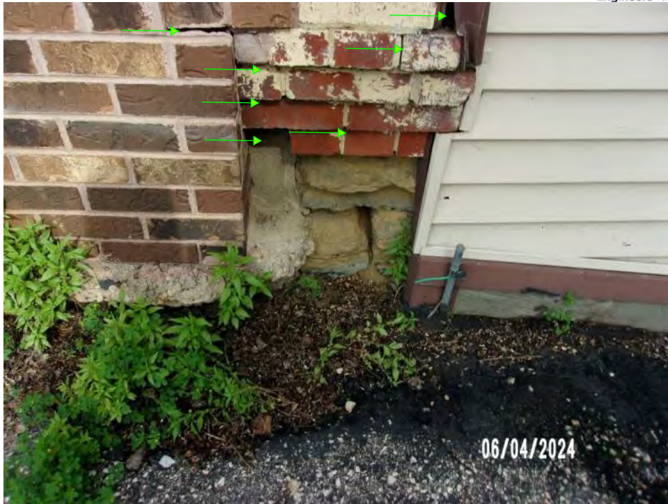
Photo 5 - Loss of mortar at the corbel near the ground on the southeast corner of the building
