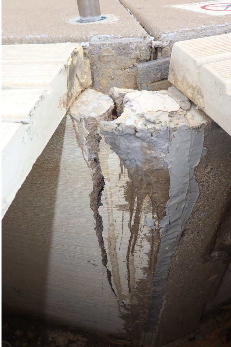
Figure 22 View illustrating cracking at south wall transition corner—outer wall
