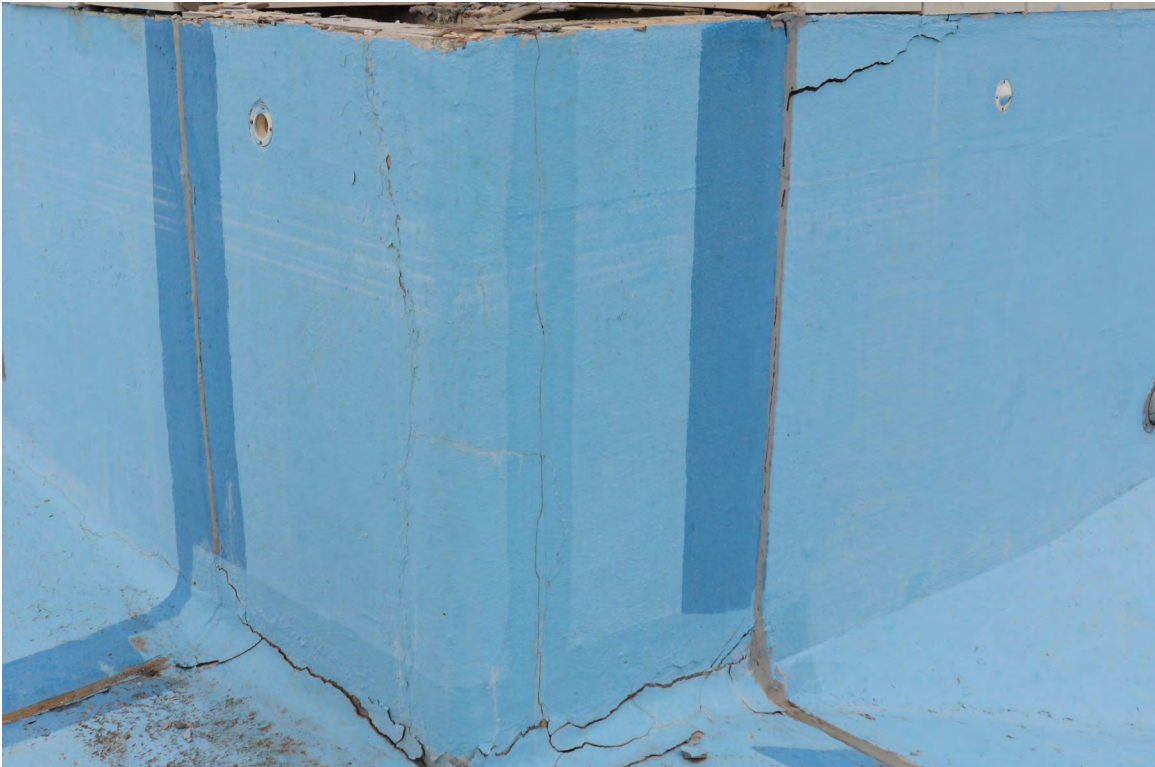
Figure 11 Close up of cracking at south end of west wall—looking north
