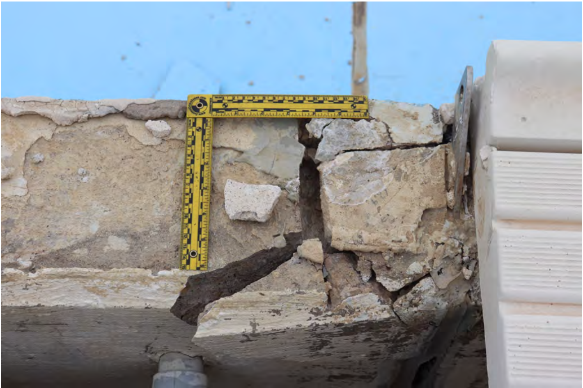
Figure 25 Close-up view illustrating cracking south of exit stairs
