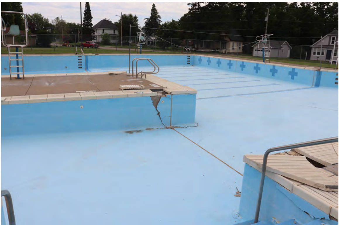
Figure 12 View illustrating east wall of slide area
