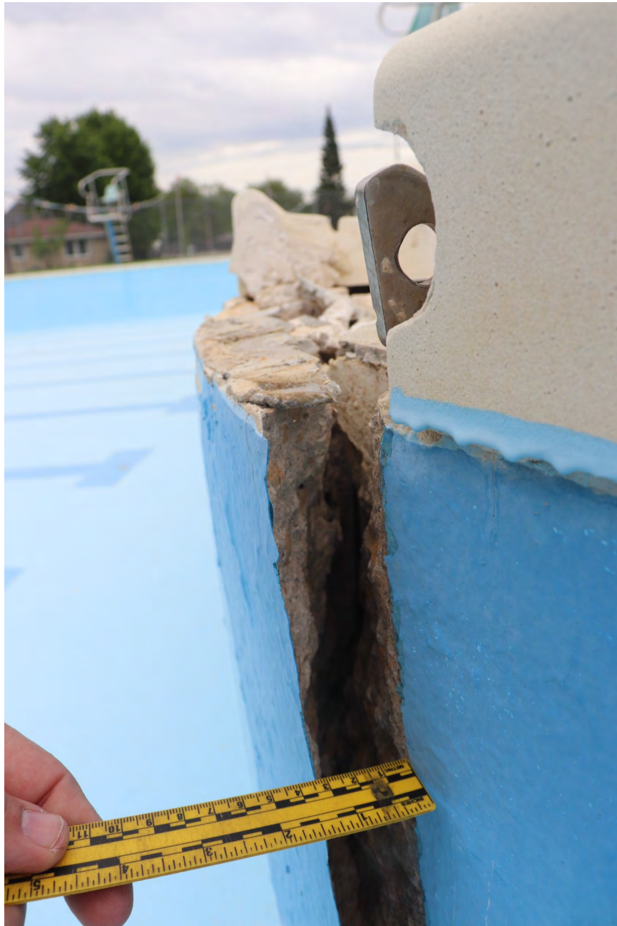
Figure 23 View illustrating shell displacement
