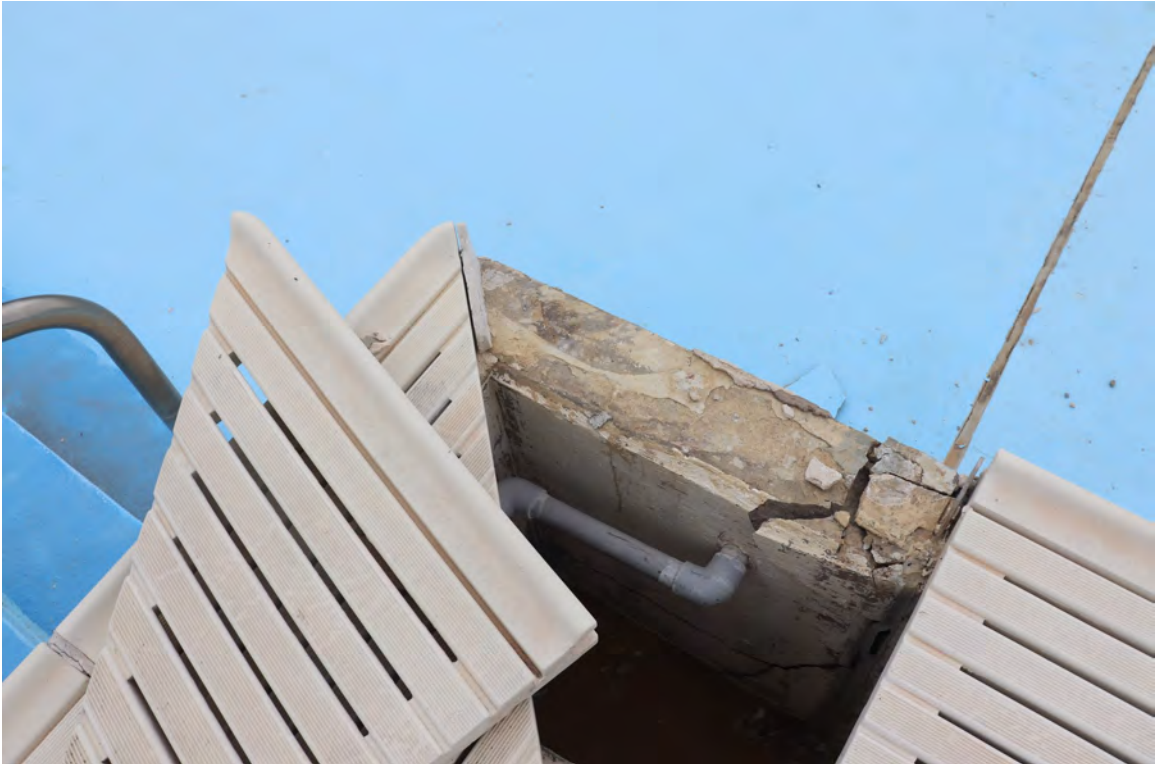
Figure 24 View illustrating inner shell wall cracking—south of slide exit stairs
