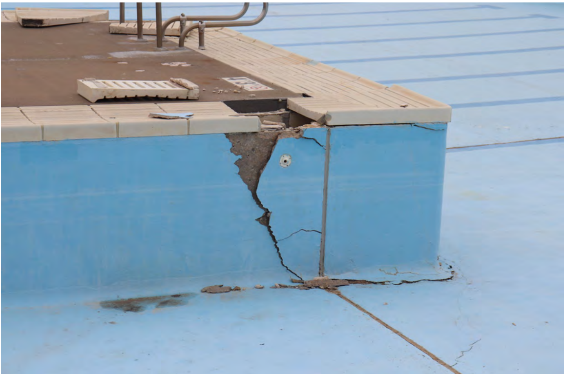
Figure 13 View illustrating cracking of pool shell—east slide area wall
